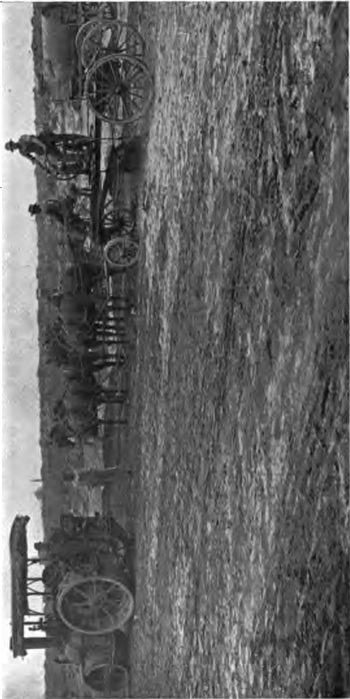
PLATE 197.—Hill View Reservoir. Spreading, Sprinkling, and Rolling of Embankment Forming Rim of Reservoir.
